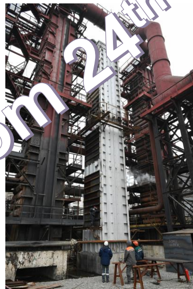
Coke oven gas cleaning plant
